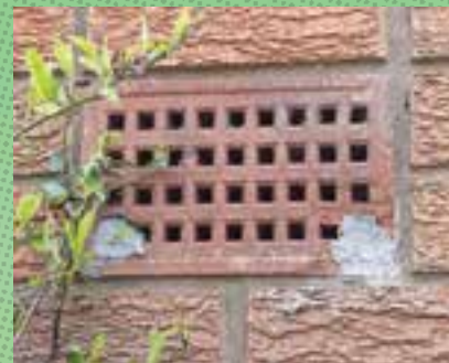
Damaged corners to an airbrick, allowing the transit of mice, are sealed with premixed mortar. The airbrick is at some height but the texture of the bricks and the presence of a shrub allow for an easy rodent ascent.
