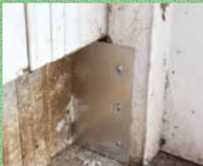
Timber frames can rot at ground level, due to being sat in rainwater. Rodents can easily chew through this rot. Proofing is achieved with an aluminium plate secured by wood screws.
