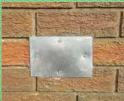
A hole left by removed waste water pipes is covered by an aluminium plate secured by screws and sealed with clear silicone.
